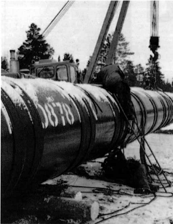
Fig. 3 — A pipeline-welding site in Russia where FAMILIARC™ LB-52U is used for joining the girth joints in freezing weather
